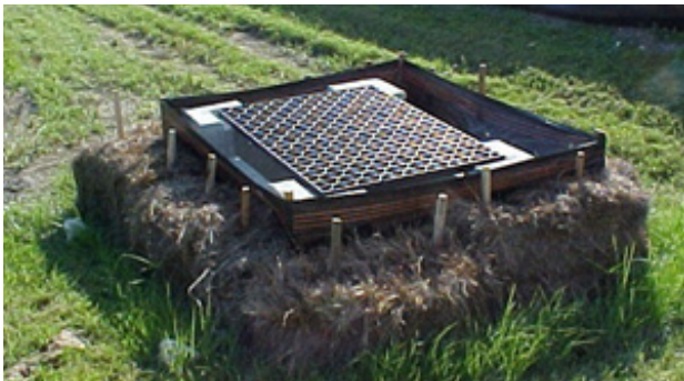
Drop Inlet Protection
