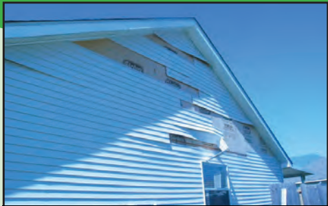
Loose and missing siding
