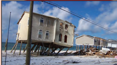
Foundation, roof, walls unsound, Multi-Family (MF)
