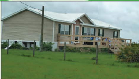
Affected Manufactured Home, skirting affected
