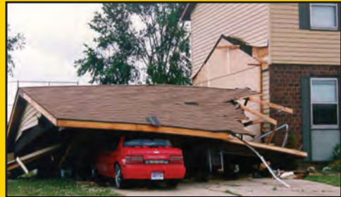
Damage to wall small breach, Multi-Family (MF)
