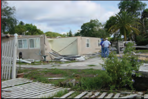
Roof & walls collapsed, Single Family (SF)
