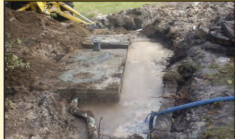
Flood septic tank damage
