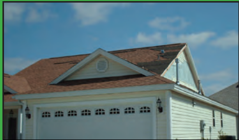
Few missing shingles, covered, no impending weather
