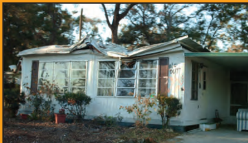
Roof partially collapsed, Manufactured Home (MH)
