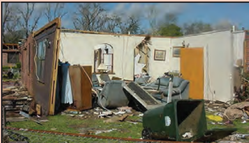
Roof gone, walls collapsed, Manufactured Home (MH)
