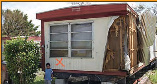
Wall coverings damaged and exposed, Manufactured Home (MH)
