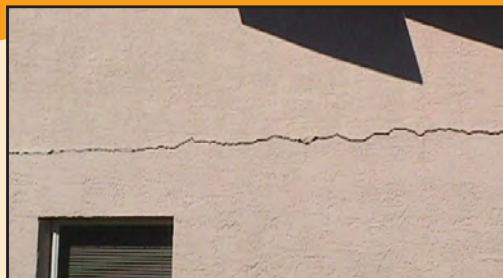
Structural cracks—roof lifted, Single Family (SF)
