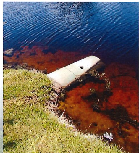
Figure 4: Exposed & damaged drainage pipe depicting the receding lake bank.
