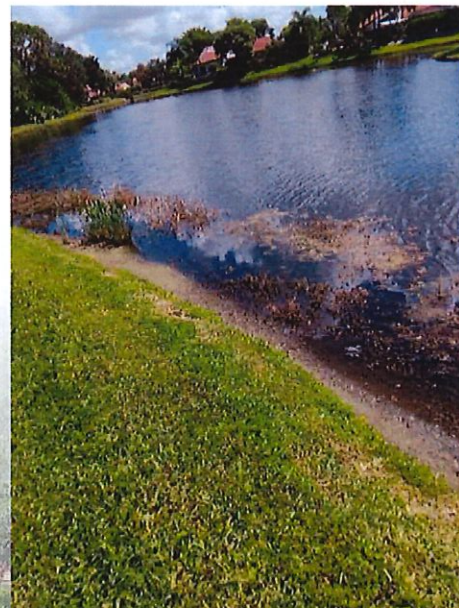
Figure 3: Erosion causing the lake bank to "slide".
