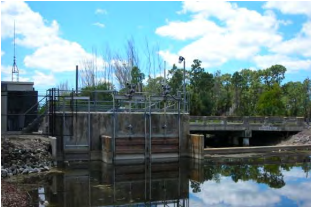
Figure 14. Upstream view of Henderson Creek Control Structure No.1 Showing Ogee Weir, Automated Sluice Gates, and Manual Sluice Gate (Photo Courtesy: SFWMD)
