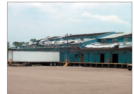
Fig. 3.39 Damaged Farmers' Market Buildings
