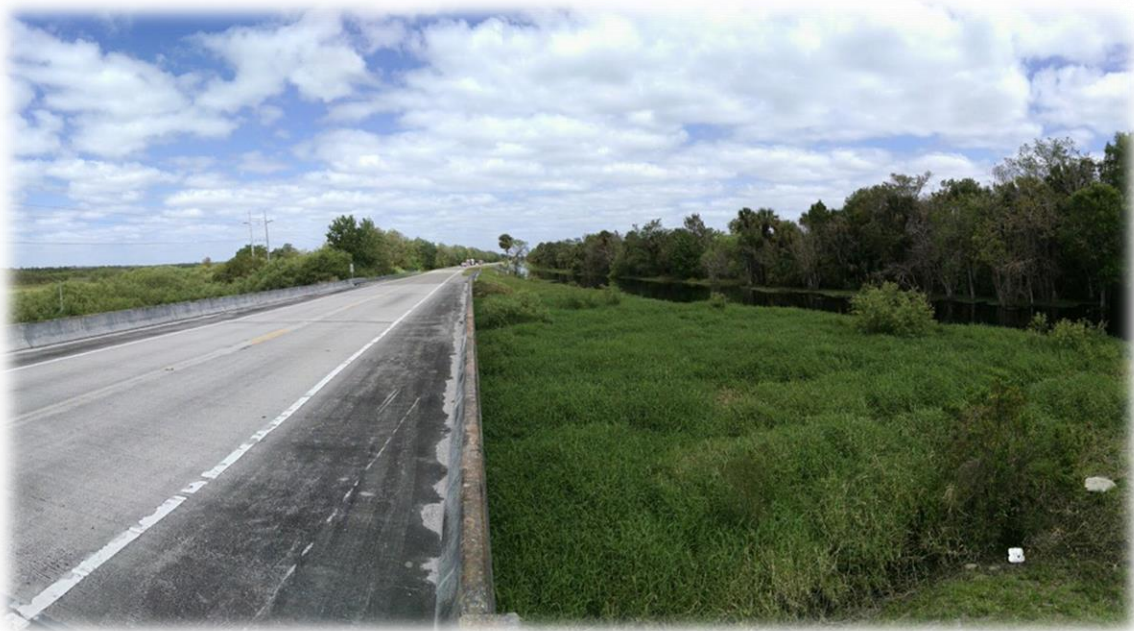
Figure 4: Looking north at third bridge north of I-75 during the wet season. Note the abundance of vegetation under the bridge
