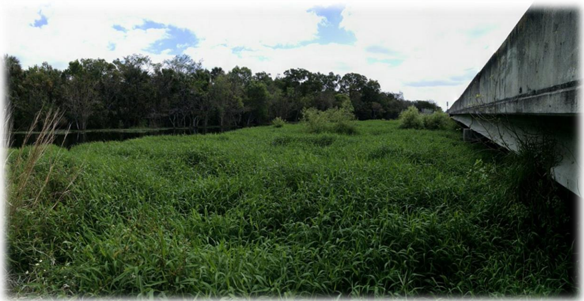
Figure 7: Even during the peak water season, water from the canal does not flow under the bridges into the Florida Panther Refuge, looking south
