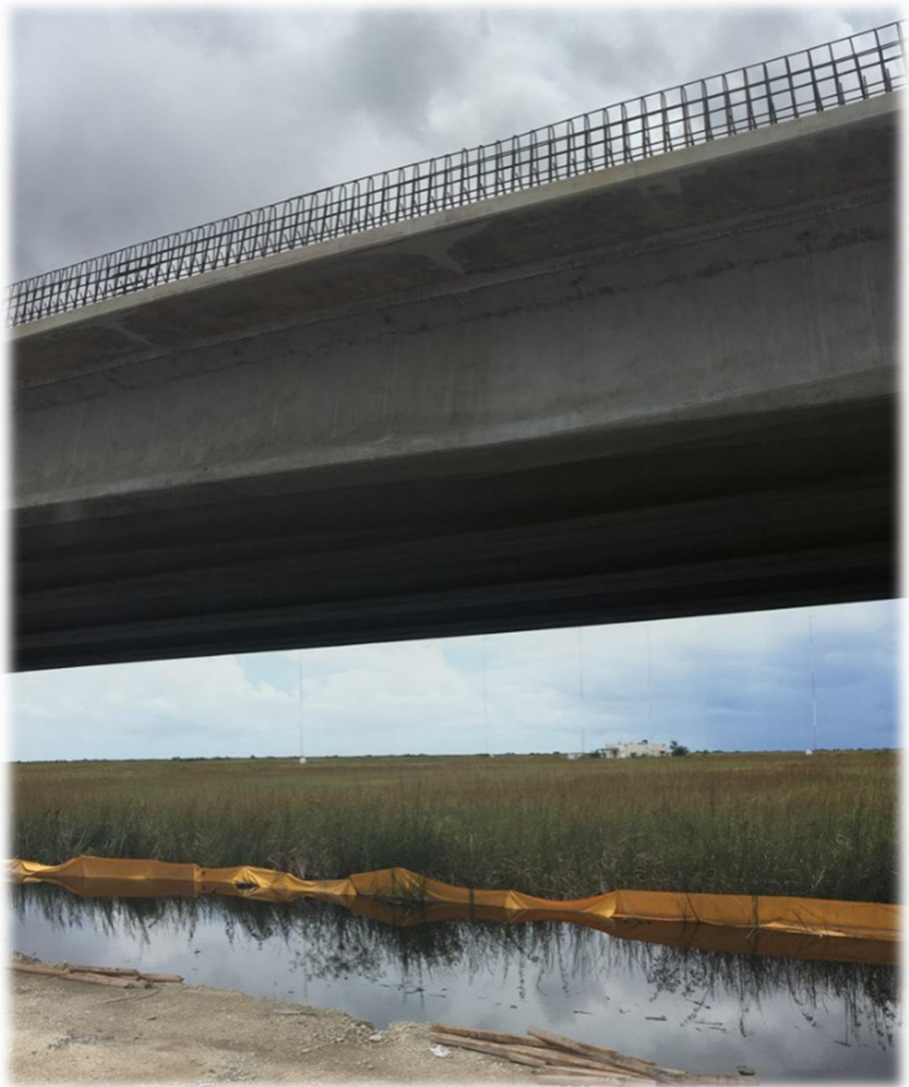
Figure 12: View of one of three new bridges being along the Tamiami Trail to help shift more water into Northeast Shark River Slough and downstream Florida Bay. Could a similar approach be championed along the SR29 road and canal corridor?
