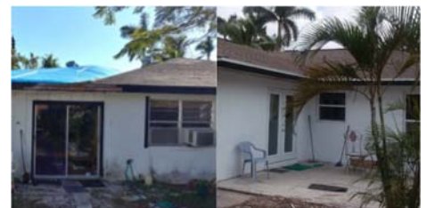
Before and after of damaged roof and porch
