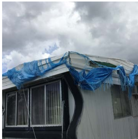
Damage caused by Hurricane Irma
