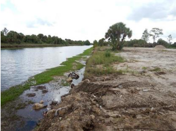
Figure 1. Absence of silt fence and soil stabilization adjacent to waterway.
