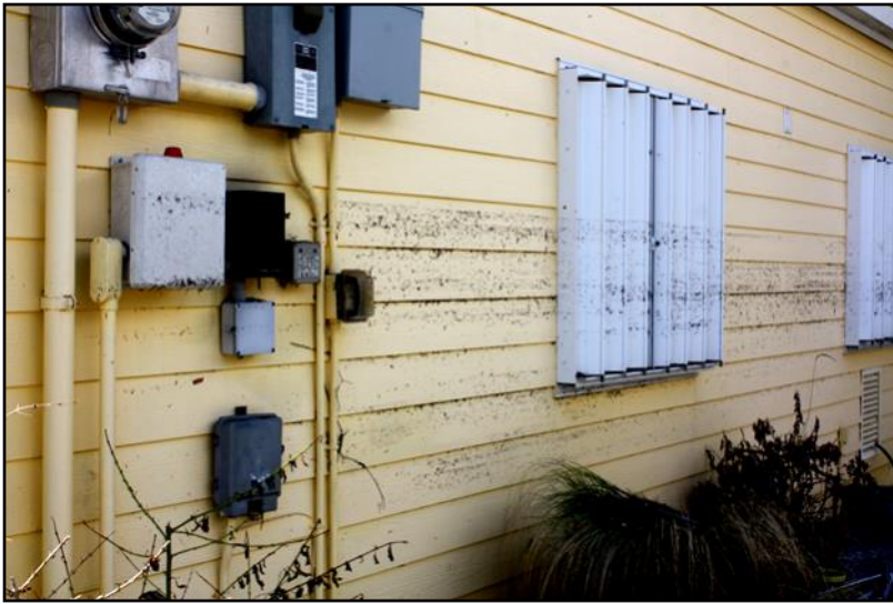
Look how high the water got on this house, well above the window
