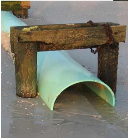
Blocked Discharge (Outfall 9)
