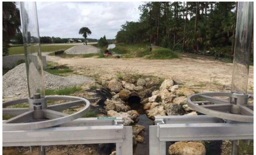
Existing canal along the east side of Wingsouth Airpark is being improved for regional flow capacity
