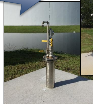
Monitor Well No. 3
