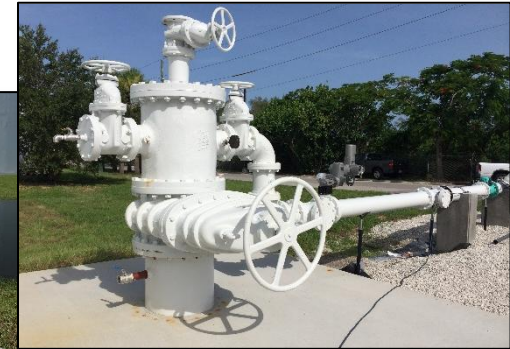
ASR Well No. 3
