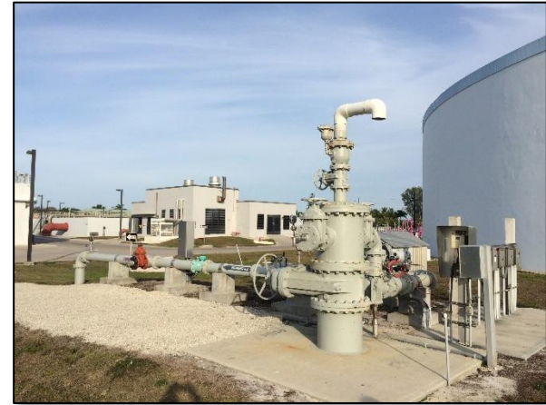
ASR Well No. 1
