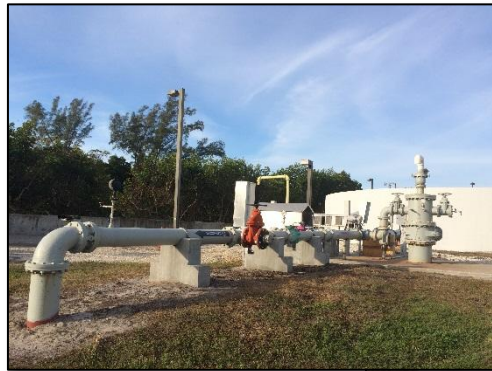
ASR Well No. 2
