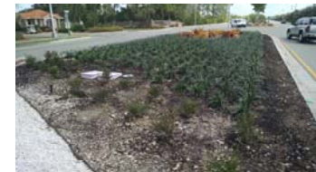
Only 2 rows of Walter's Viburnum installed instead of several rows
