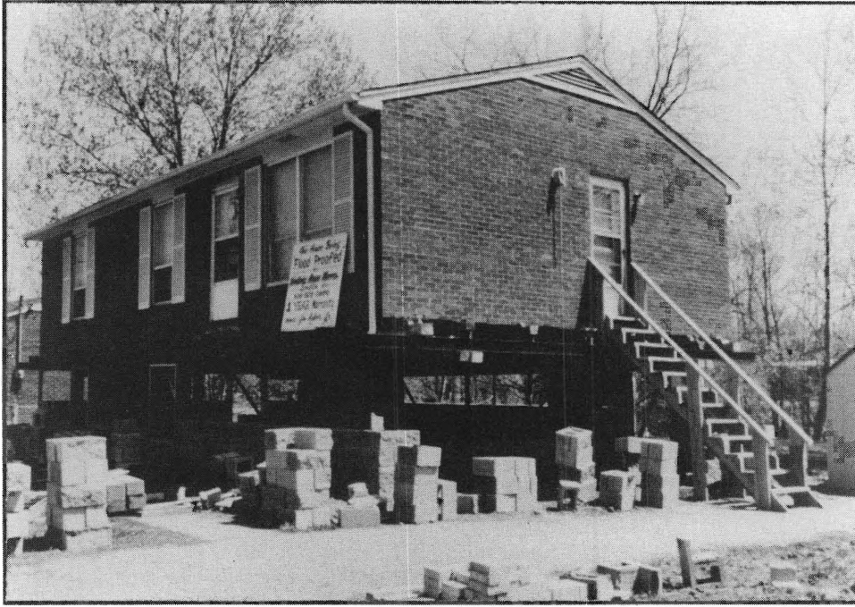
Figure 4: Example Of A Home Raised With The Brick Veneer In Place — During Construction.
