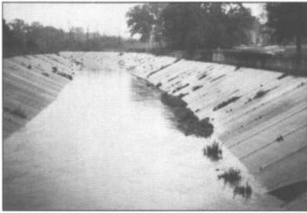
Storm drainage is a significant problem in many large urban areas, particularly if development has been rapid and not well planned. Drainage systems must be designed to handle infrequent, but potentially catastrophic, events.
