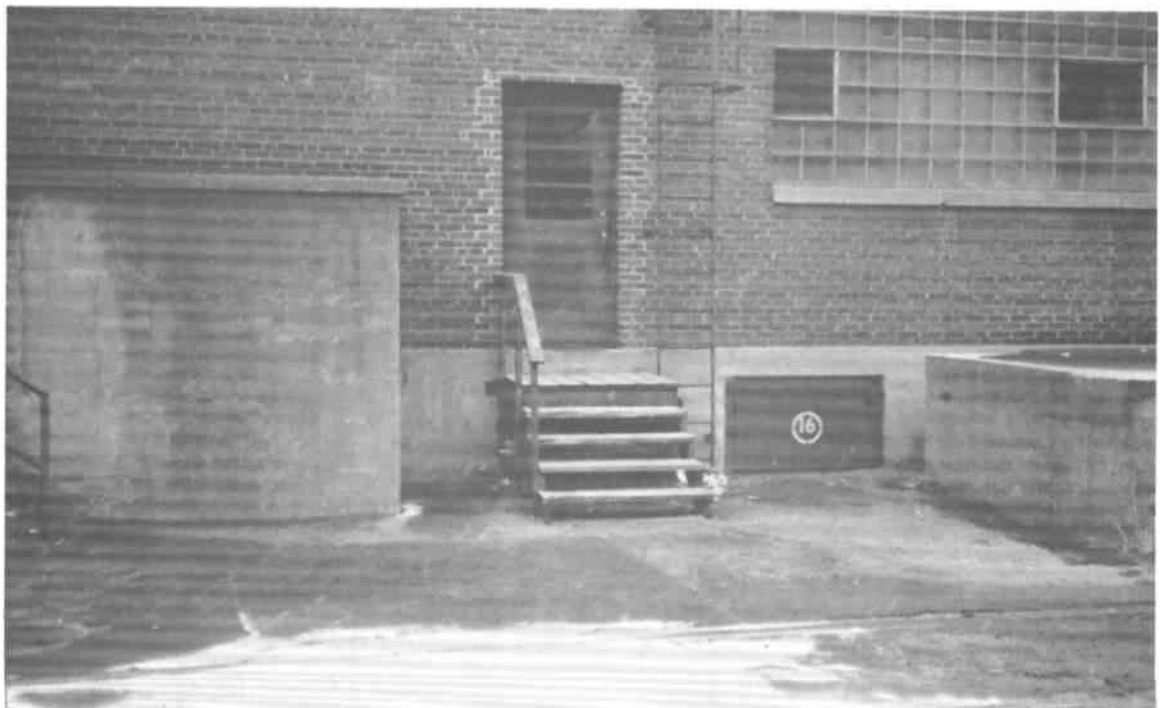
Flood shields are maintained in place over seldom-used openings.
