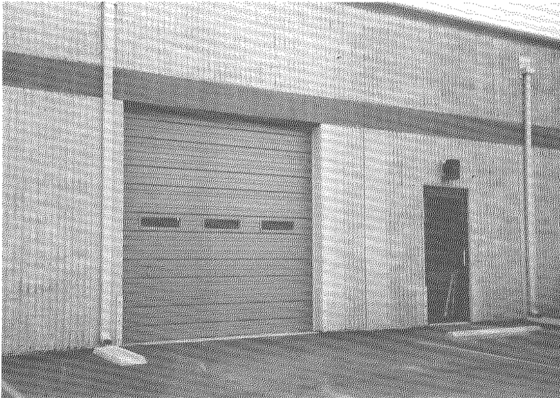
Floodproofing requires installation of 18 flood shields to protect 8 vehicular entrances and 10 personnel doors.
