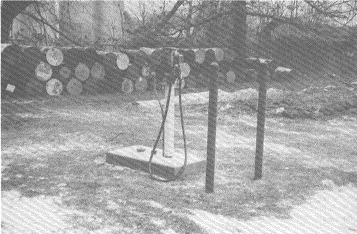
Floodproofed on-site gasoline pump to provide fuel for portable pumps and other equipment.
