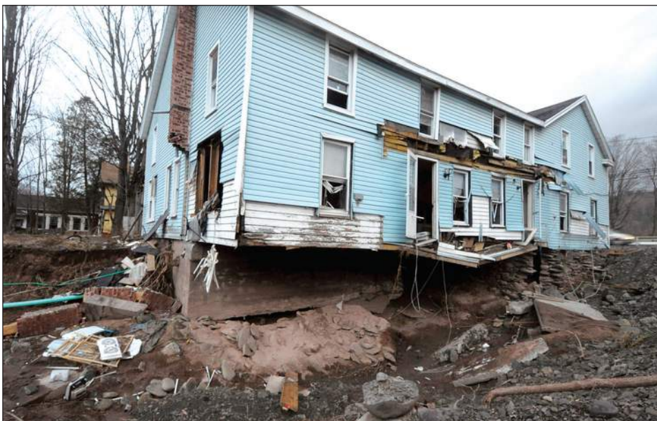
Figure 3 13. Many homes in the Town of Prattsville, NY, were slated for demolition during the recovery effort following Hurricane Irene.
