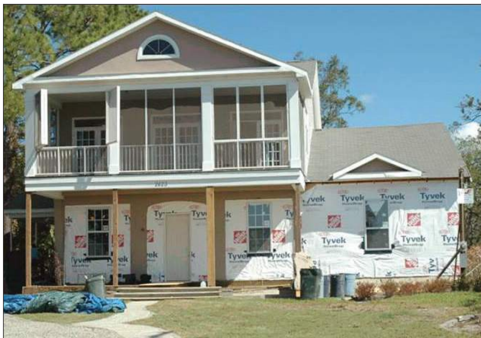
Figure 2-1. This home in New Orleans was inundated by 4 feet of water during Hurricane Katrina.
