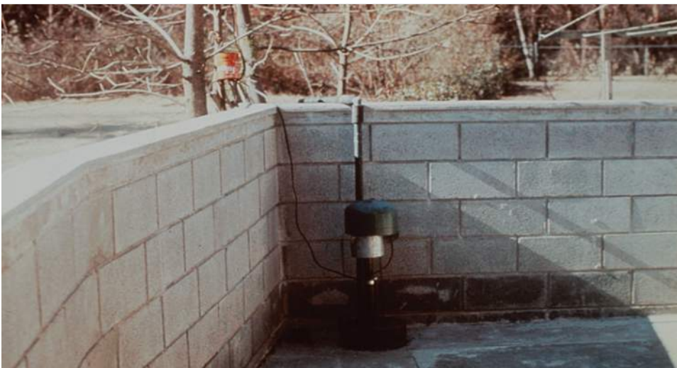
Figure 8-6. Small patio floodwall with sump pump.
