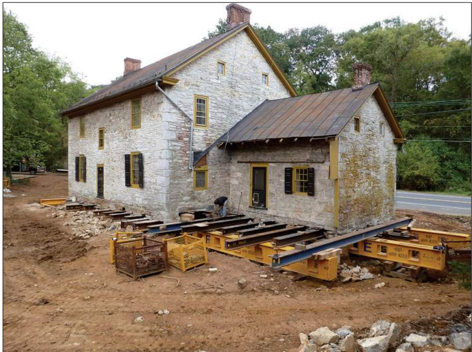
Figure 6-4. Beams supported by cribbing are placed at critical lift points (photo courtesy of Wolfe House Movers).
