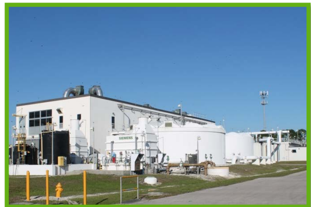
Exhibit 2-9: NCWRF Sludge Processing Facility
