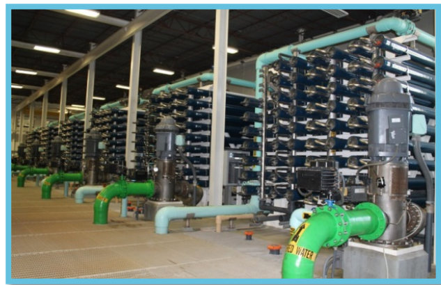
Exhibit 2-2: NCRWTP LPRO Treatment Skids
