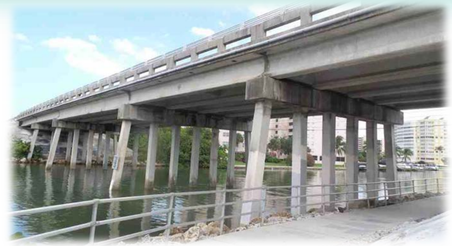
Photo 4 - Delnor Wiggins Bridge (Bridge No. 030149) that carries Bluebill Avenue over the Vanderbilt Channel was built in 1969.
