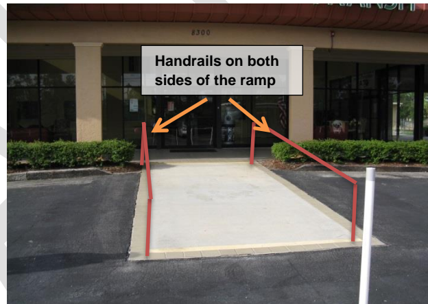
Incompliant entrance ramp slope
