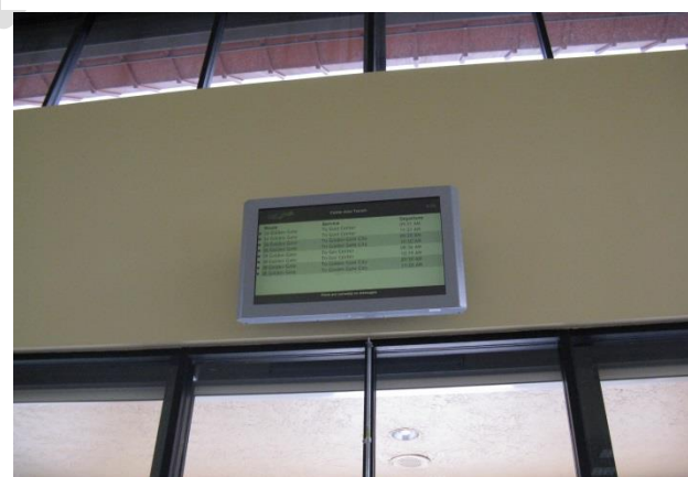
Incompliant character heights
