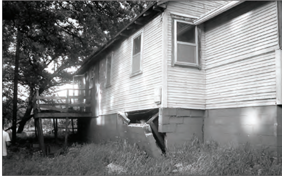
Figure 2-8. The walls of this basement in Iowa failed because of the pressure exerted by water and saturated soil.
