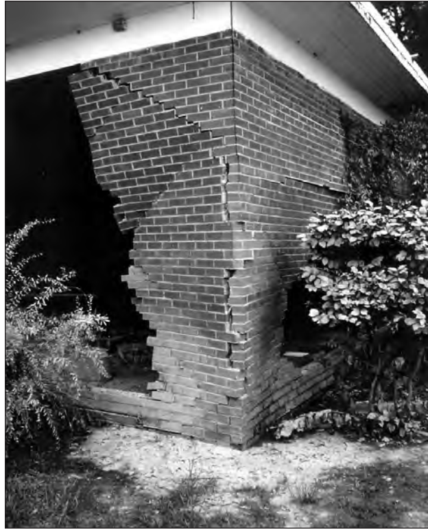
Figure 2-11. Moving water can cause walls to collapse, as illustrated by this riverine flood damage in Georgia.
