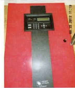
•Goodwill-Roberts Center •Immokalee, FL •Fire Alarms
