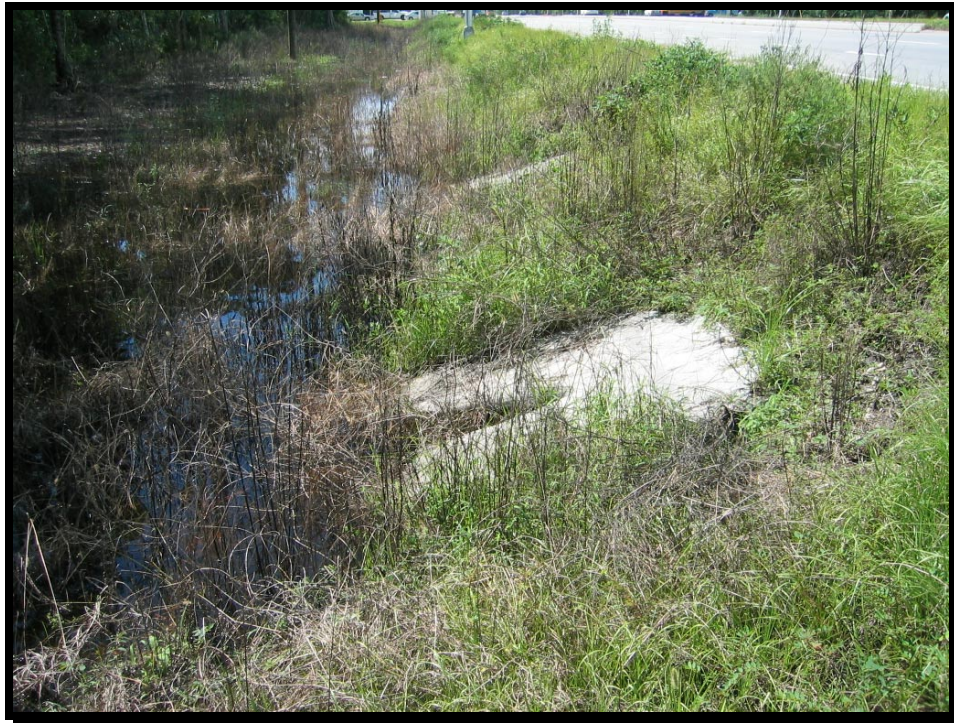
Photo 6. Two 18-inch culverts maintain some degree of hydrologic connection with lands to the north of Pine Ridge Rd.
