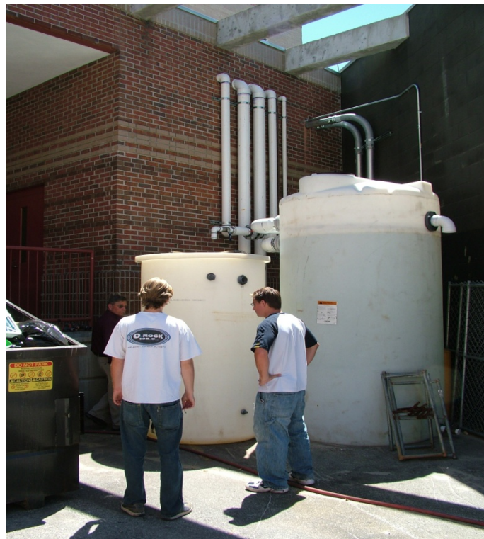
Figure 3.4-2 Example of Above-Ground Industrial Cistern Storage
