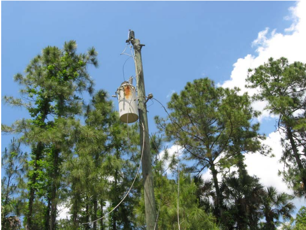
View of pole-mounted transformer along southern property boundary
