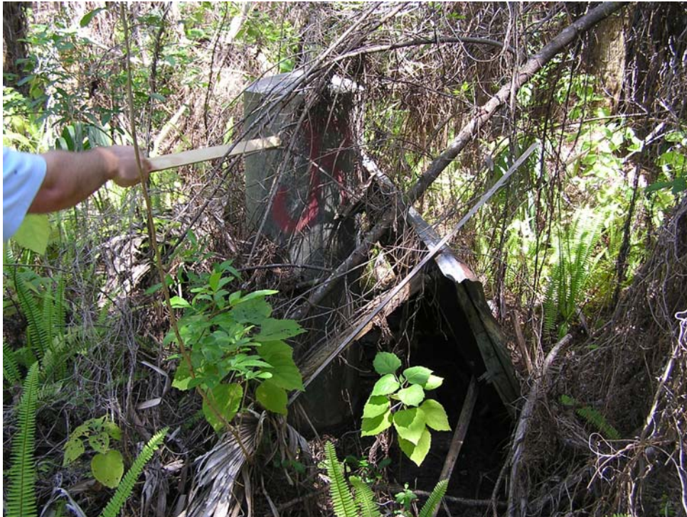
Water heater adjacent to trailer (southwest portion of property)
