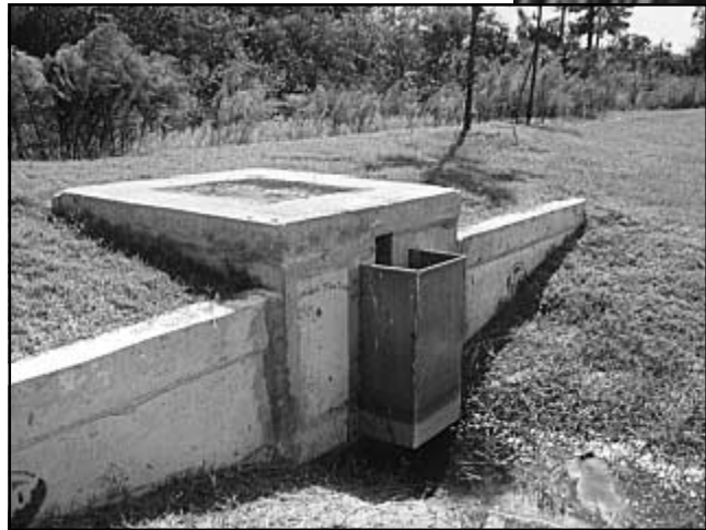
▲ Outflow Control Structure
