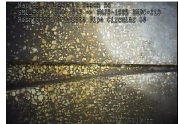
Joint Separation/Signs of Pipe Sinking
