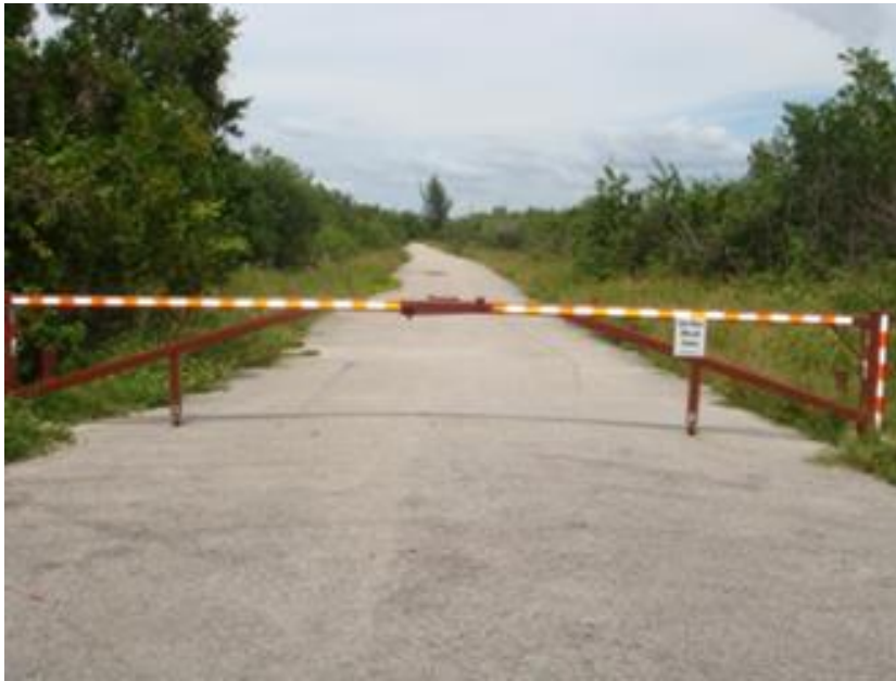
Heavy-duty gate installed at the intersection of Curcie and San Marco Rd.
