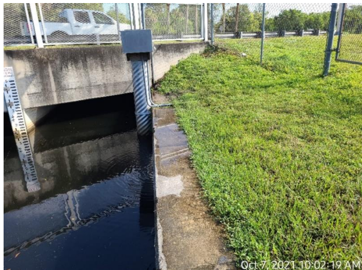
Figure 6. Sewage leak from 8" pressurized main line entering Gordon River at Golden Gate Pkwy.
