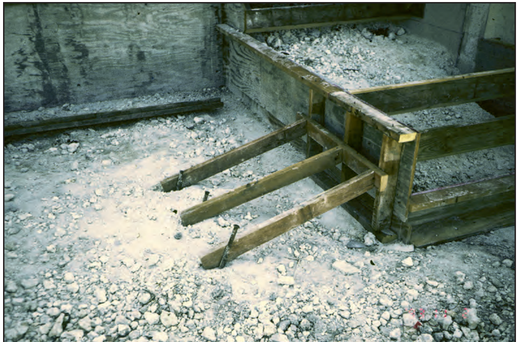
Figure 33 Wood framing for a new concrete staircase that will provide access to the elevated floor.
