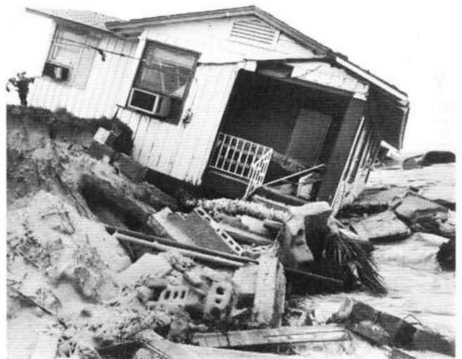
Figure 2.3. Erosion Caused This Foundation to Collapse.
